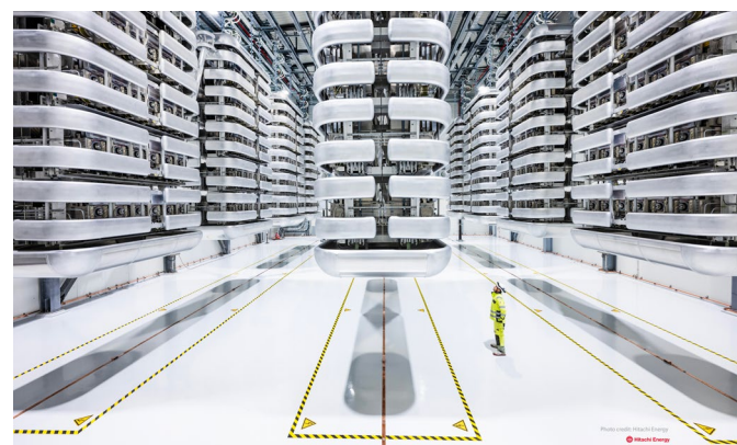
Picture: inside a converter station, photo credit: Hitachi Energy
